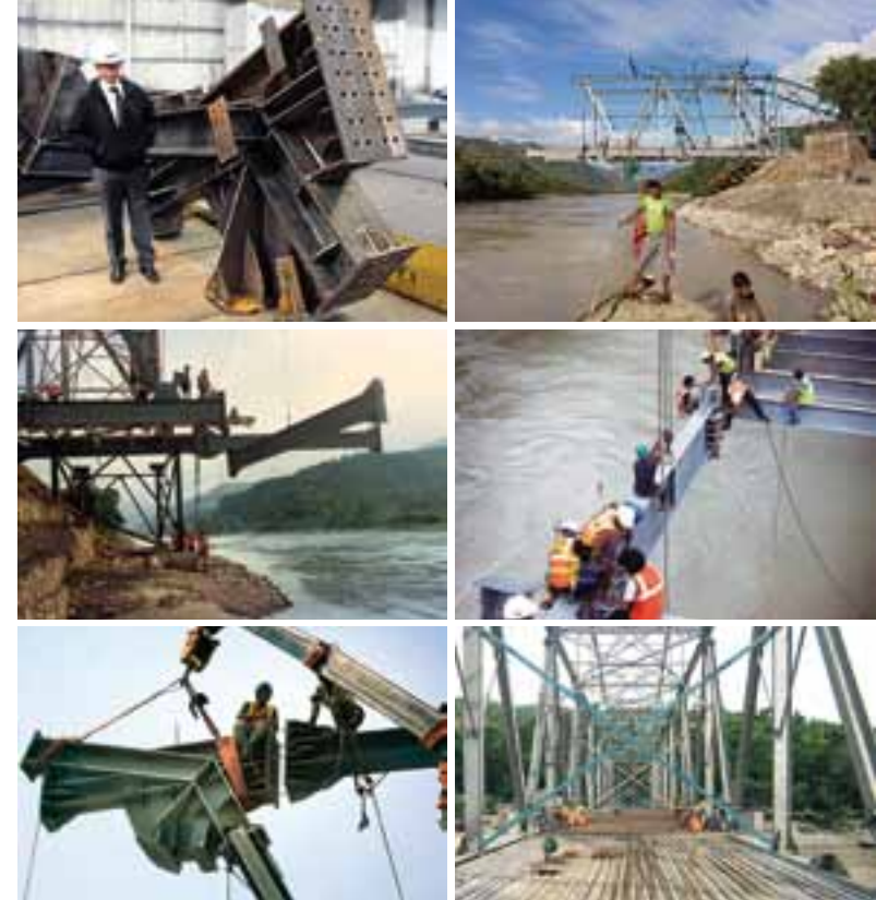
Above and right: images of the bridge during construction Bottom right: the completed Arun Bridge
