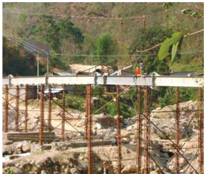
Figure 2. The lower chord being built on old pylons resting on gabions, on aerial ropeways.
