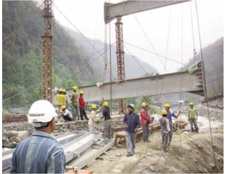
Figure 3. Kalika workers sling in heavy members by hand suspended from aerial ropeways.
